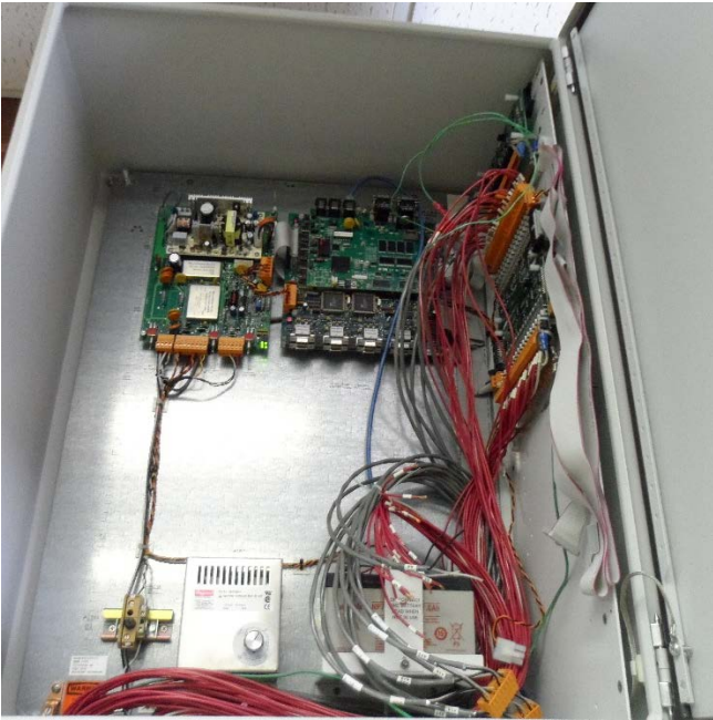
Control Building Survalent Equipment
